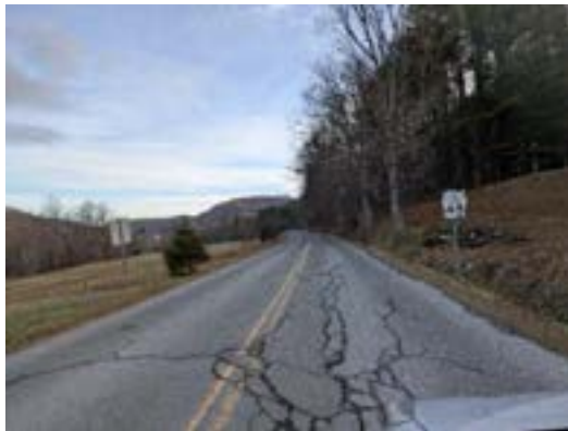
Existing pavement condition on Pomfret Road
