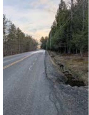
Ditch along Pomfret Rd
