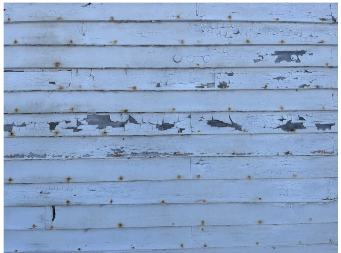
Deteriorating Wood Siding
