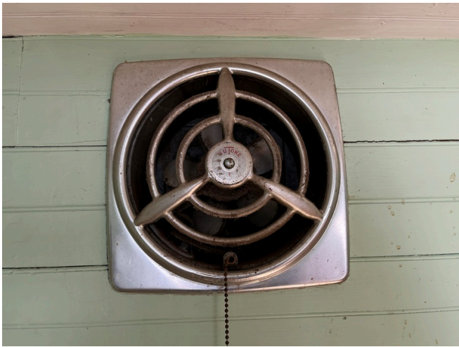
Kitchen Ventilation System
