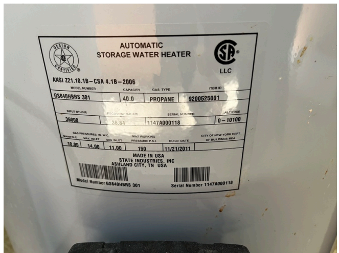
Propane DHW Tank Nameplate
