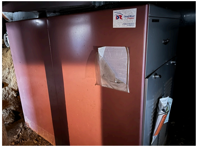
Oil Burning Furnace
