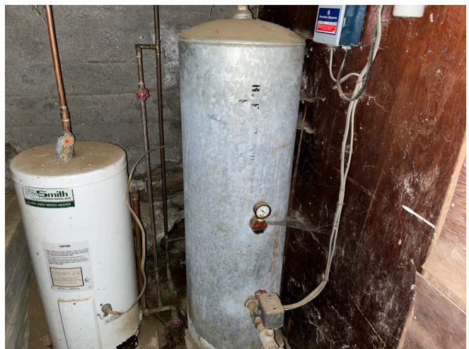
DHW Storage Tank
