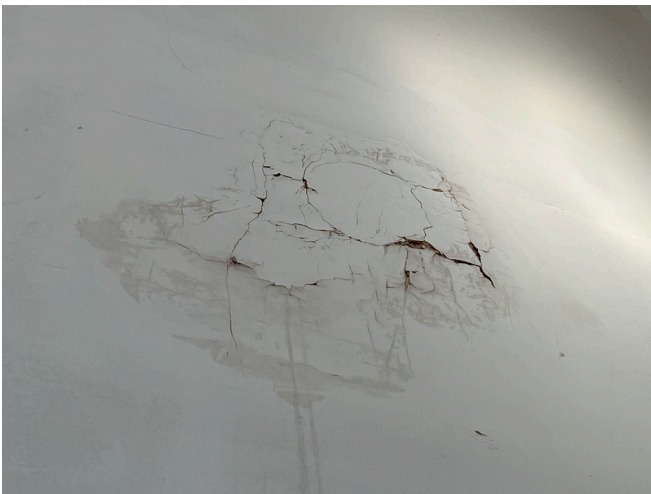
Deteriorating Wall from Chimney Moisture
