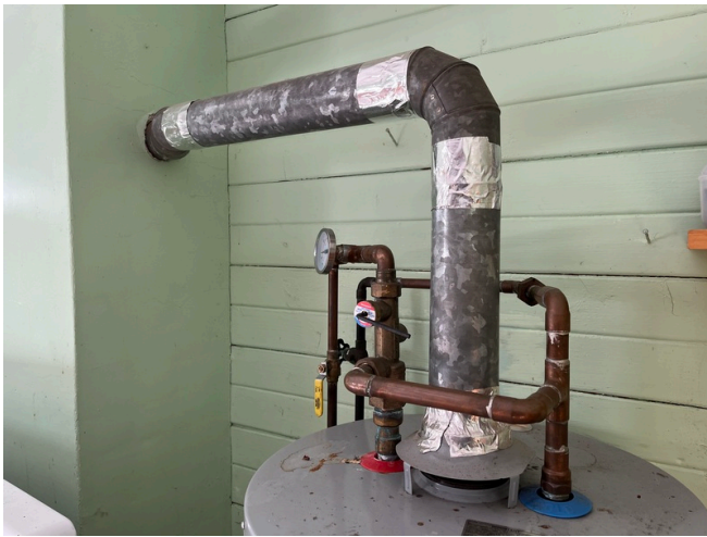
Un-Insulated Distribution Lines
