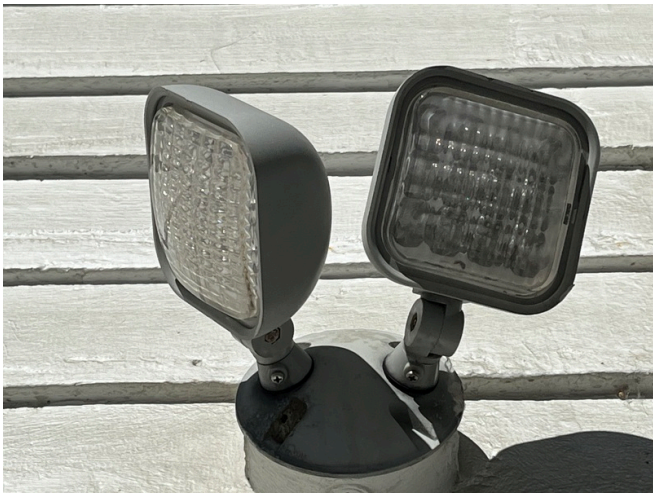
Typical Exterior Flood Light Fixture
