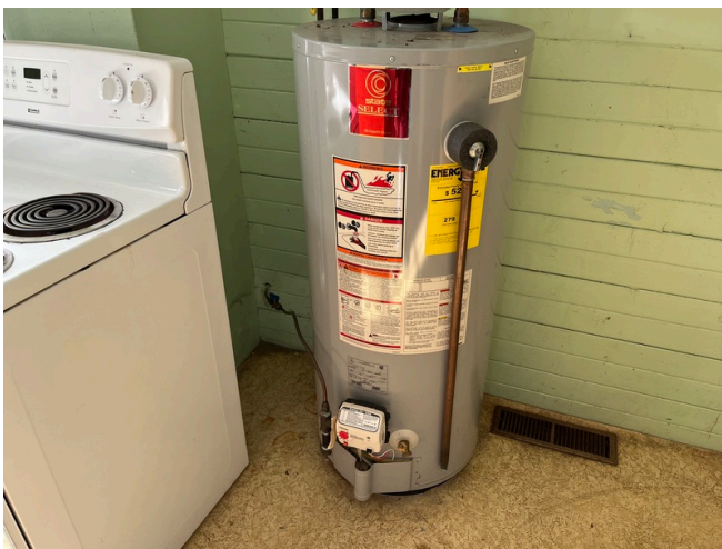
Propane DHW Tank
