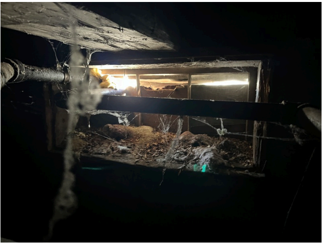
Basement Air Sealing Opportunity
