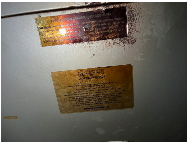
Oil Burning Furnace Nameplate
