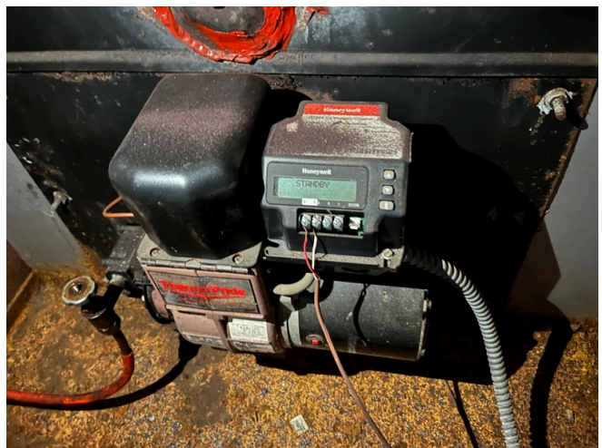
Oil Burning Furnace Control System
