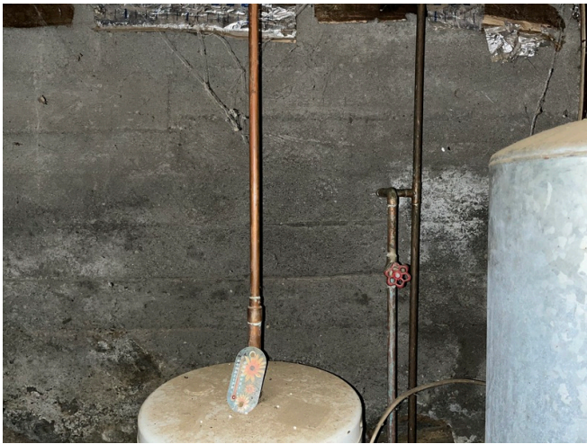
Un-Insulated Distribution Line
