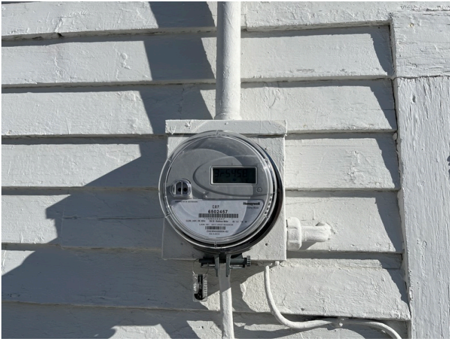
Building Electric Meter
