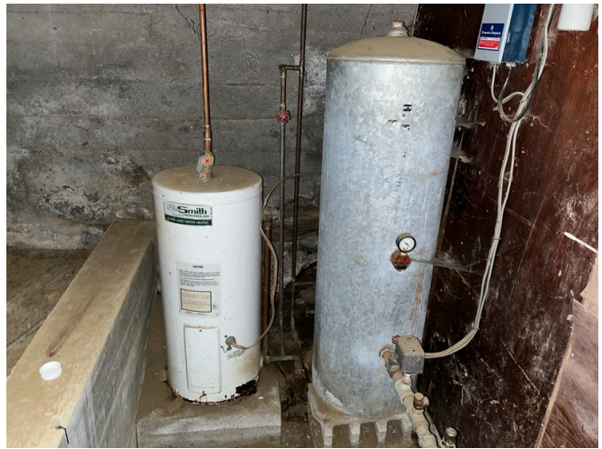
Electric DHW System
