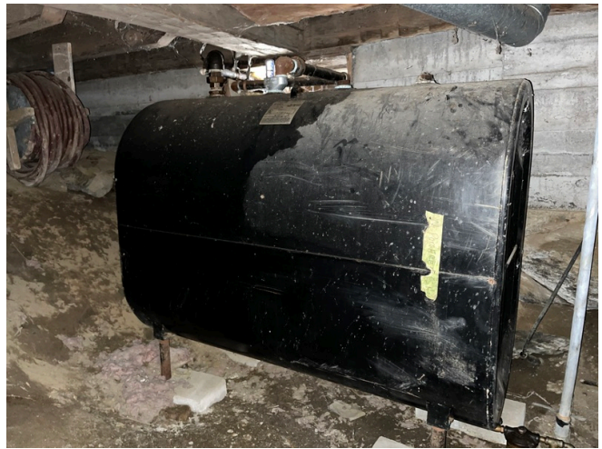
275 Gallon Oil Tank
