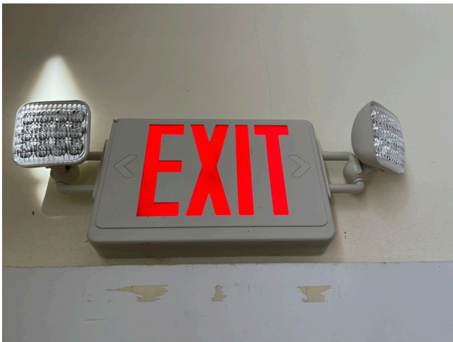
Typical Exit Sign
